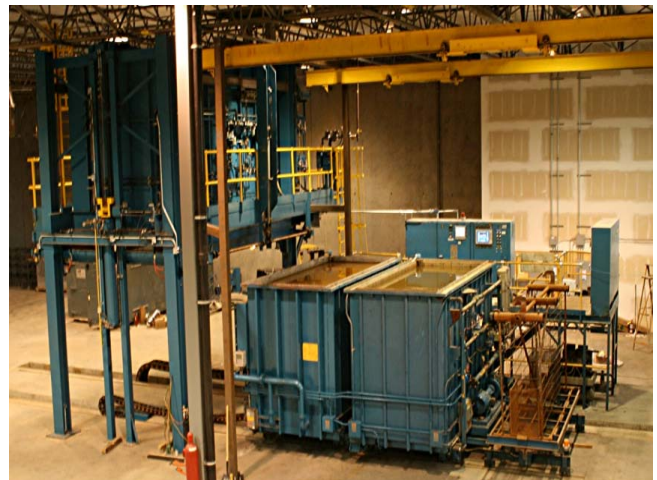
The furnace shown installed at Pyrotek
