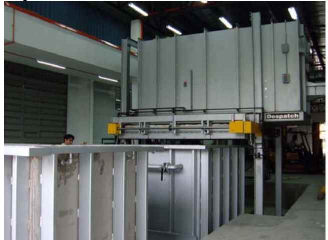
Figure 4: All major components installed and connected. (Furnace, Mobile Quench Tank and stationary rinse tank)
