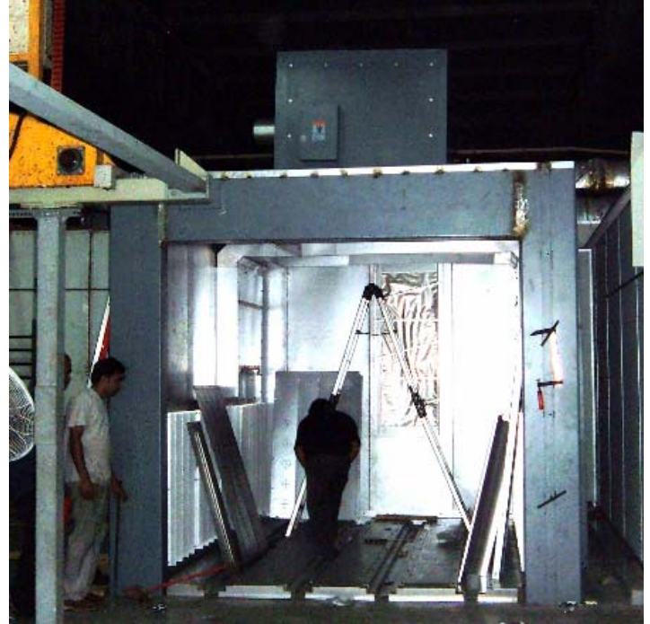
Figure 11: The supply and return duct installed and the heater box placed in the proper position.
