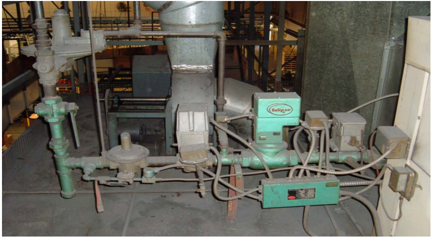
The picture shows the old gas train.
