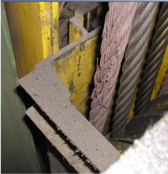
Picture show cable in the hoist.
